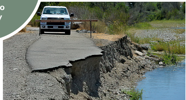
▲ 2017 storm damage along the Arroyo Mocho in Livermore.
